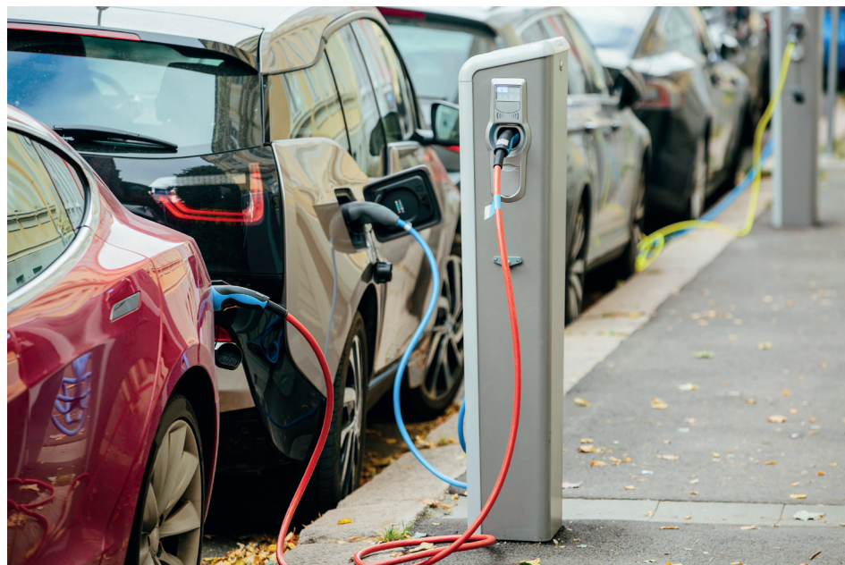
Figure 7 Chargepoints situated close to the kerb
