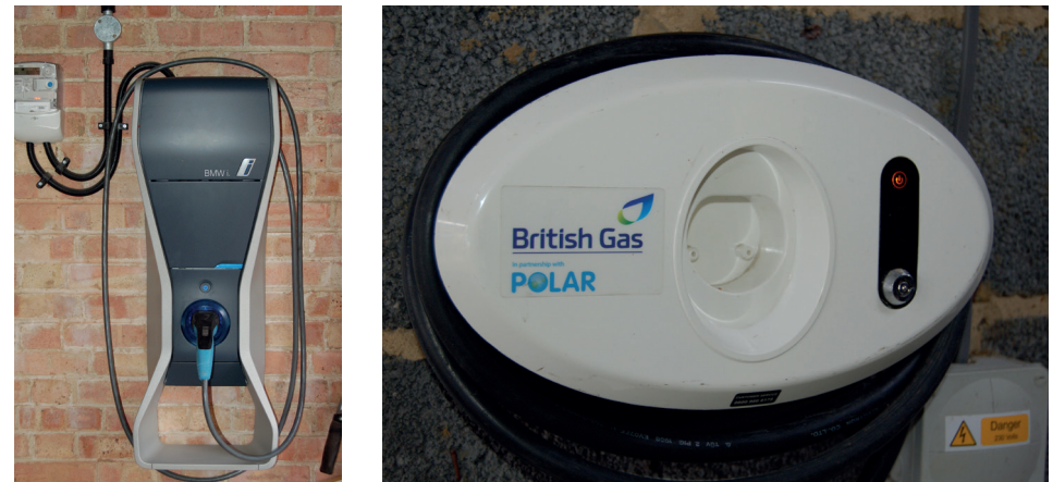
Figure 4 Typical residential chargepoint installations
