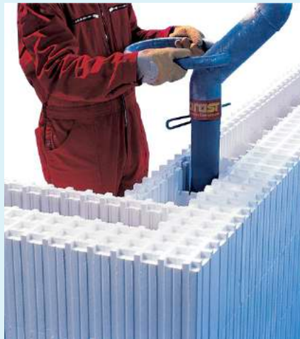
Hollow blocks of insulating material are stacked to create the mould for structural concrete walls
