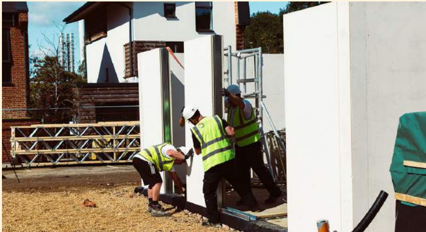
Project Etopia demonstration home, Watford, 2019, uses 'Hyper SIPS' high performing structural insulated panels, which include steel
