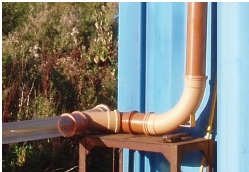
Photograph 4.4 Test facility - Soil stack connection to the drainage system
