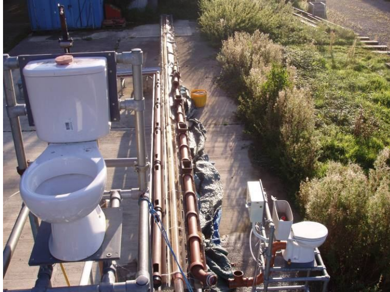
Photograph 4.1 Test rig – Layout
