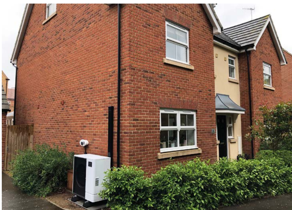
Figure 6 The external unit of an air-source heat pump (ASHP)
