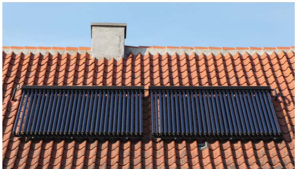
Figure 3 Solar thermal (hot water) tubes
