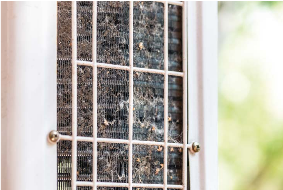
Figure 14 Blocked ASHP outside unit
