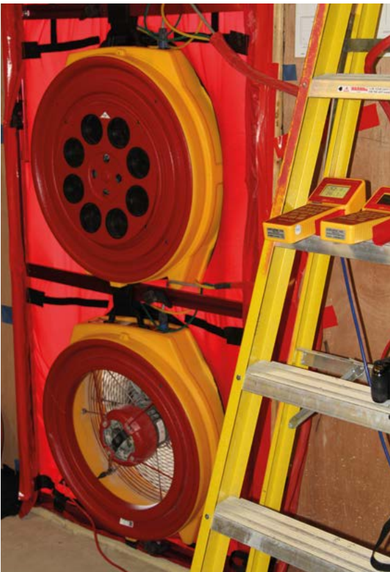
Figure 4 Examples of quality assurance processes during construction: photographically recorded key details (Top); air leakage testing (Bottom).
