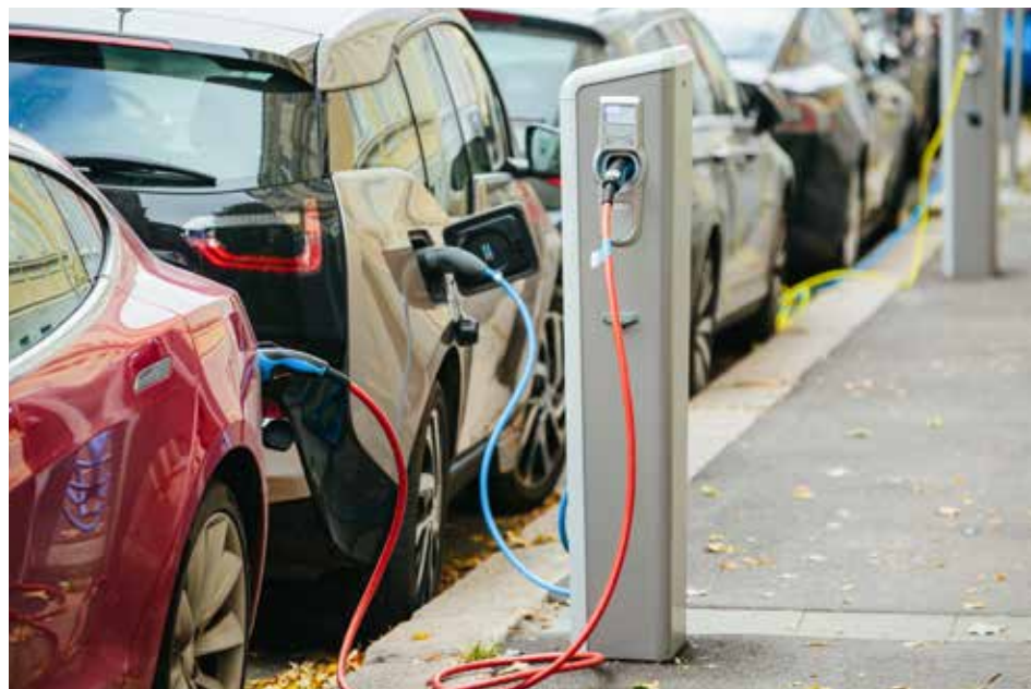
Figure 7 Chargepoints situated close to the kerb
